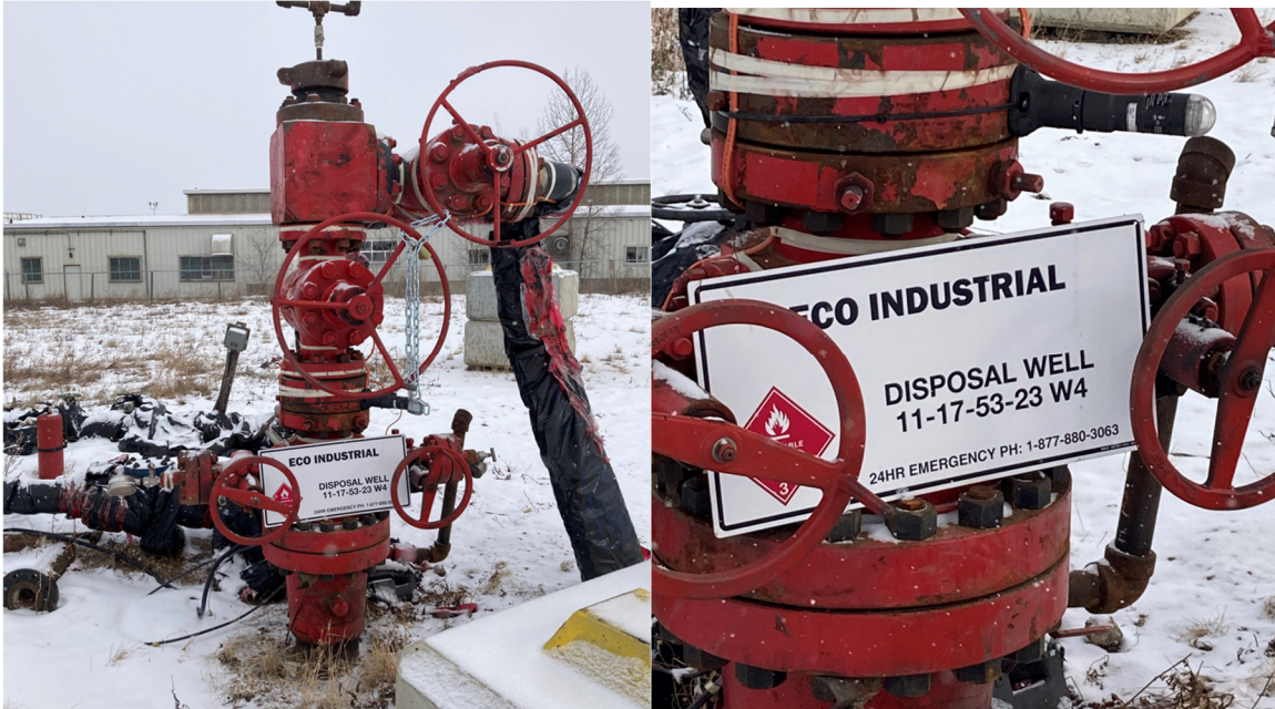
11-17-53-23 W4M Securement of Wellhead c/w Sign & Emergency Number
