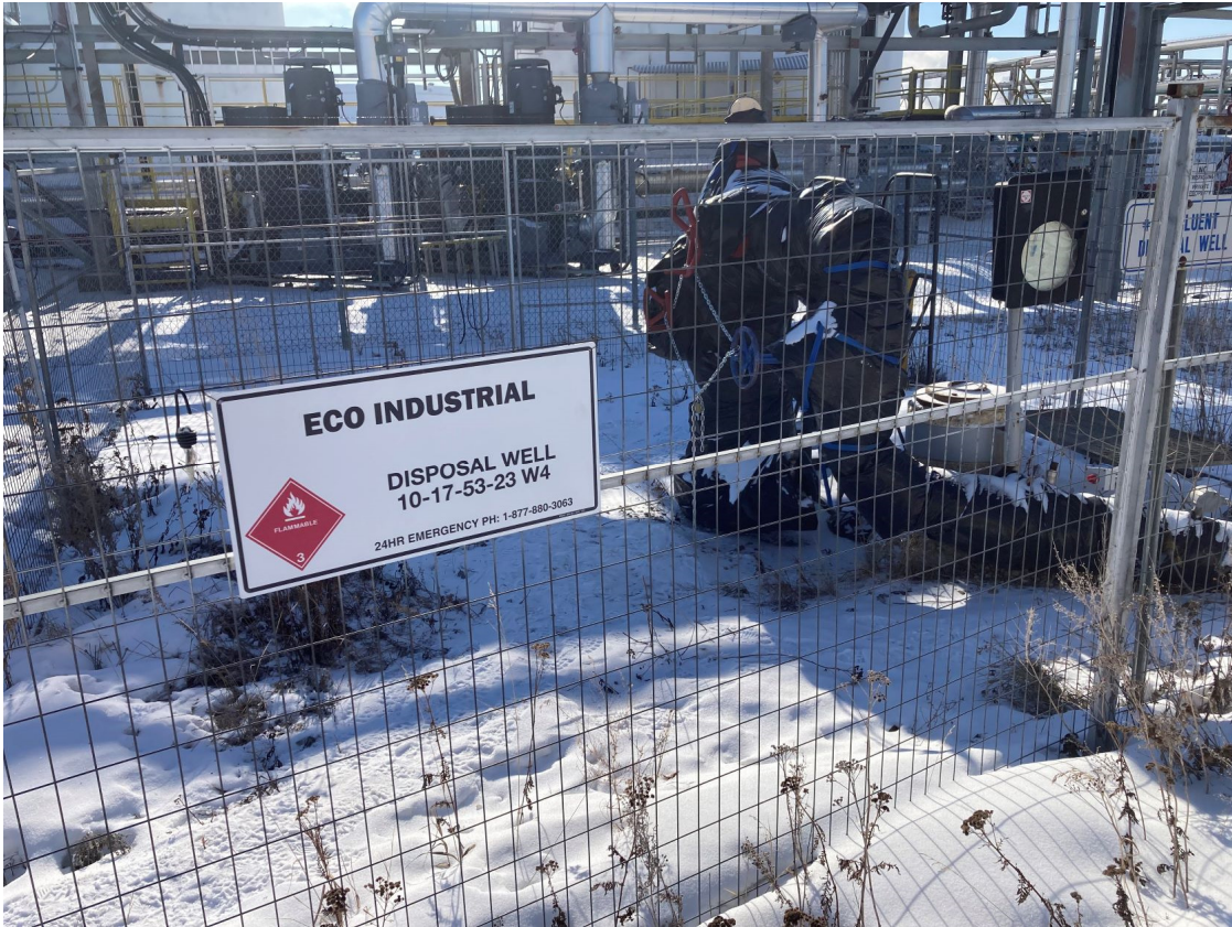
10-17-53-23 W4M Securement of Wellhead c/w Sign & Emergency Number
